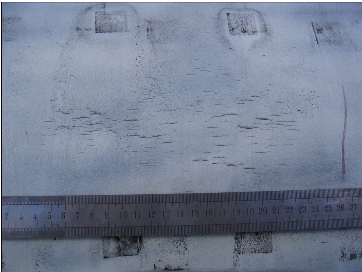
Figure 1-2: Presence of SCC on a pipeline surface as detected by MPI.
