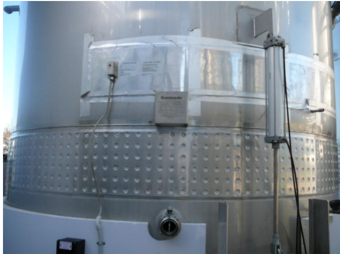
Figure 8. Heating Pad installed before bring covered by insulation at Whitebox Winery
