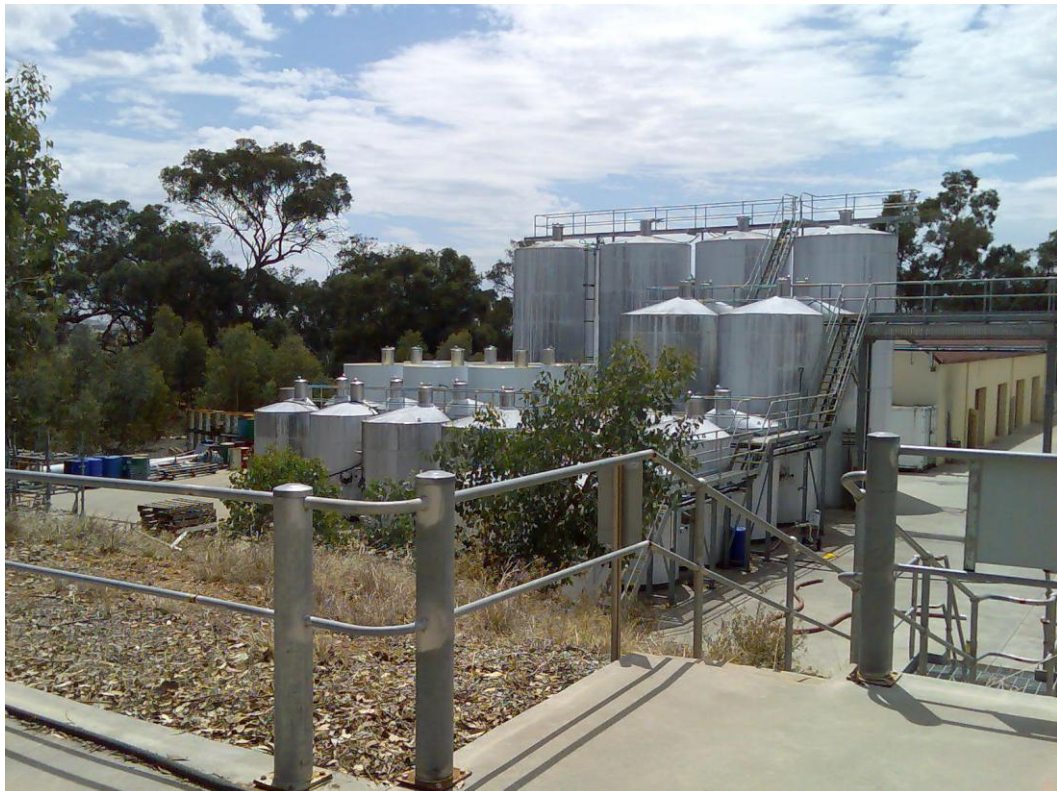
Figure 5. "The Tank Farm". External storage tanks at Whitebox Winery
