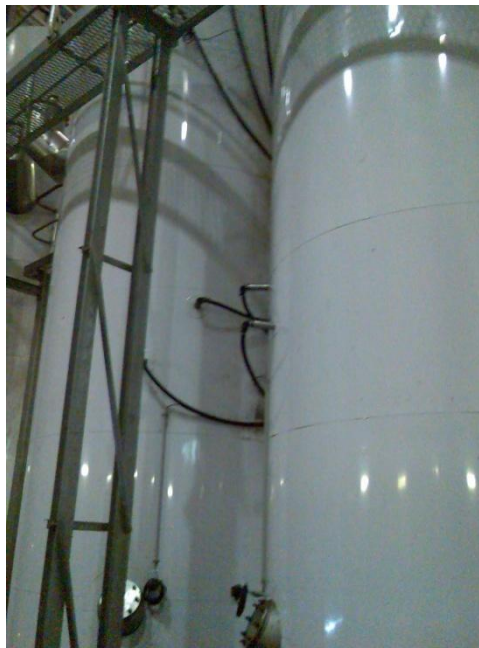
Figure 7. Cooling lines attached to vessels at Whitebox Winery
