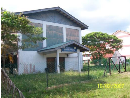
Source: Author Photograph 17: Abandon Community Hall at Pos Iskandar Date Photograph Taken 10 th February 2007
