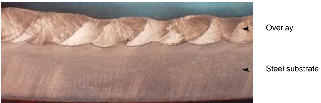
Figure 4.8: Cross-section of WeldoverlayA spool showing the preferential wear of the weld beads at specific locations having a lighter appearance. The sample has been etched in acid ferric chloride.
