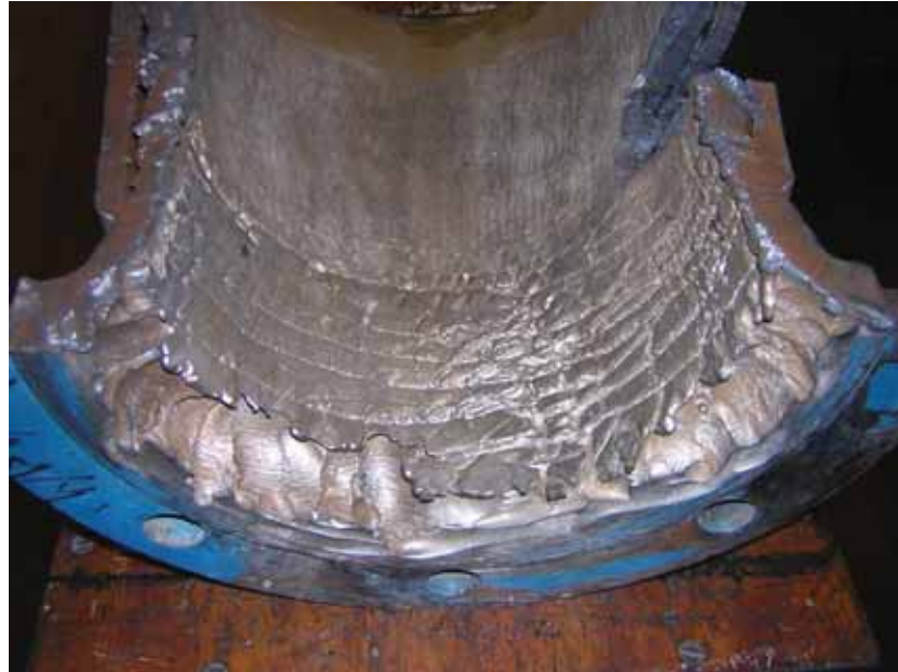
Figure 4.7: Photo of the entry section adjacent the flange of the WeldoverlayB trumpet spool. The image shows the loss of hardfacing material and the wear of the steel substrate.
