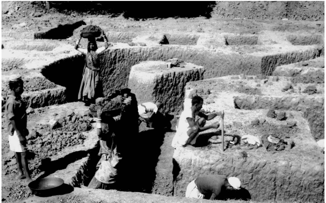
Fig. 7.40. Construction begins at the IIM site in Ahmedabad, 1964. (Source: Publications Department, Indian Institute of Management.)
