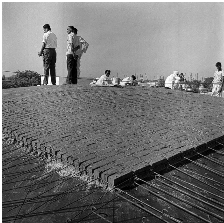
Fig. 7.58. Construction photograph, NID brick shell. (Source: NID Archives, National Institute of Design, Ahmedabad, India)
