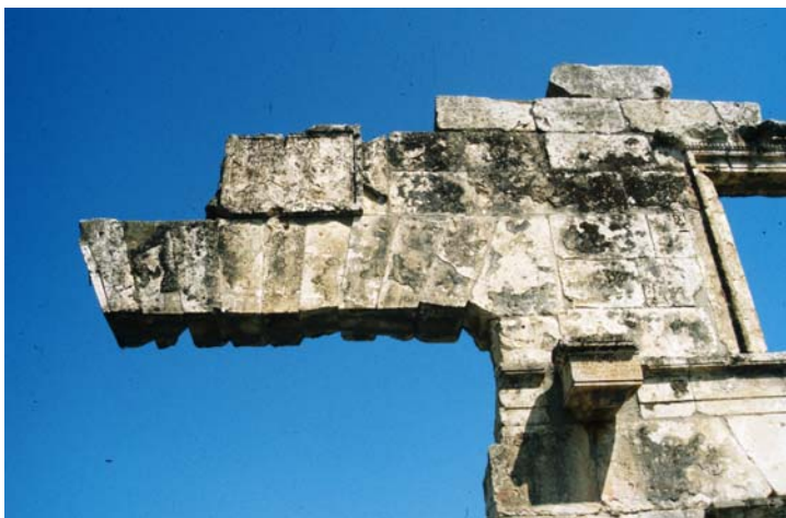
Fig. 60. Apamea: portion of a Roman stone arch in danger of collapse. (Author: 2000)
