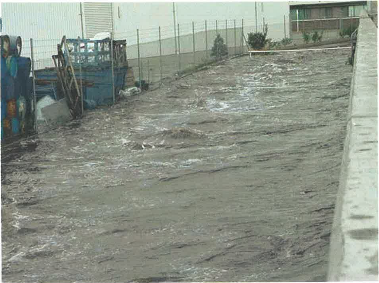
Figure C.5 Keswick Creek overflowing at Mile End, 25 January 2001
