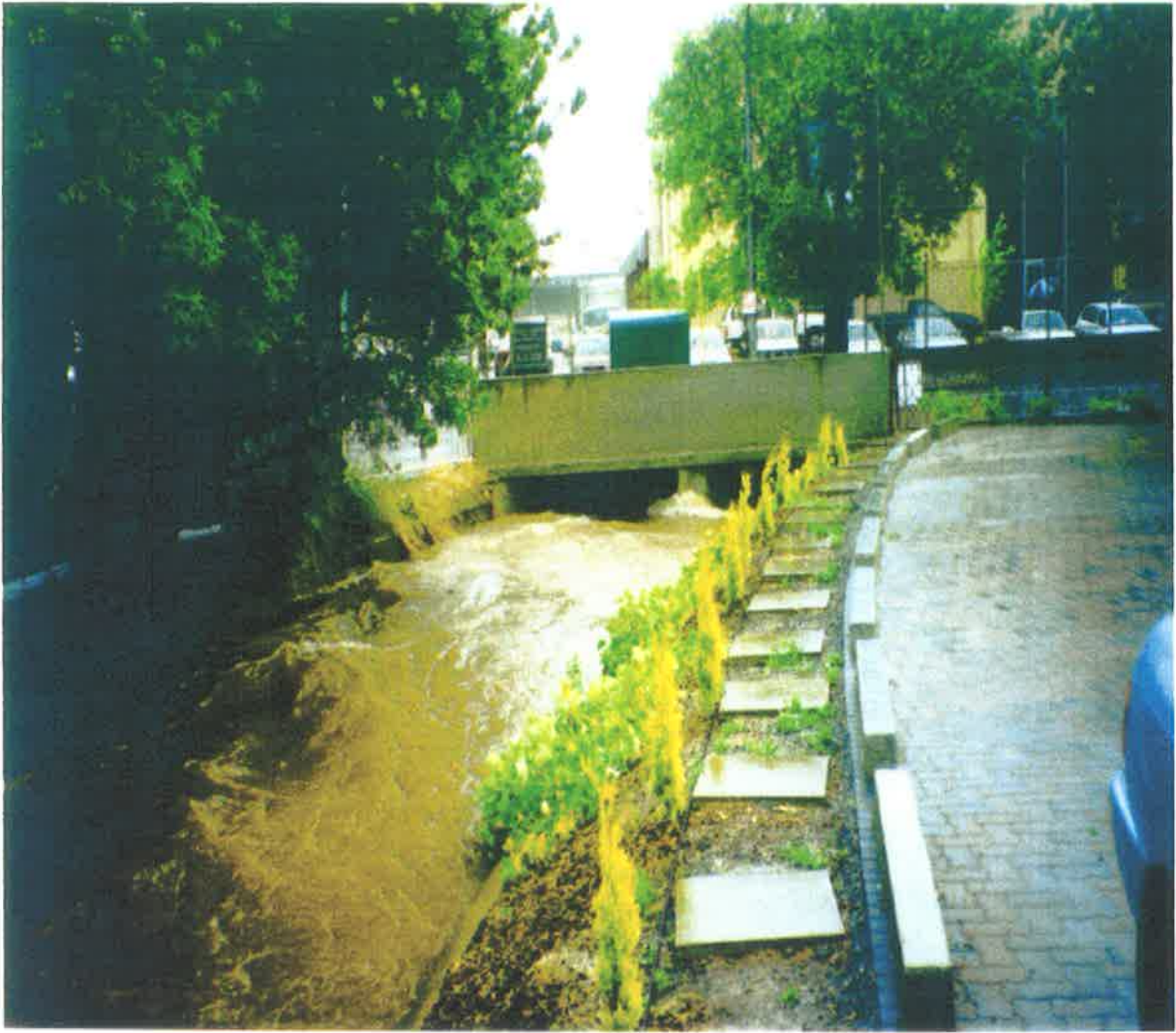
Figure C.7 Keswick Creek at the entrance to the Showgrounds Tunnel, flood of August 1999. Note: Peak flood level reached the level of the roadway.
