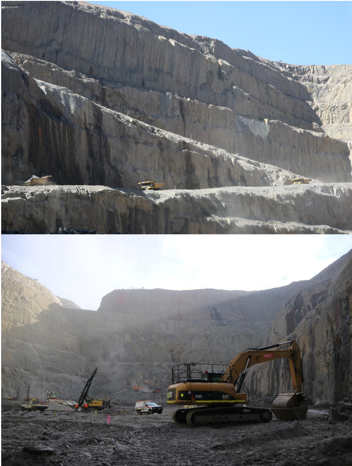
Appendix Figure 1: The Kanmantoo Mine in full operation, April 2018, 172 years after the first workings. Top: East haul road, facing ESE. Bottom: Excavation and drilling operations with the morning sun rising over the pit, facing S.
