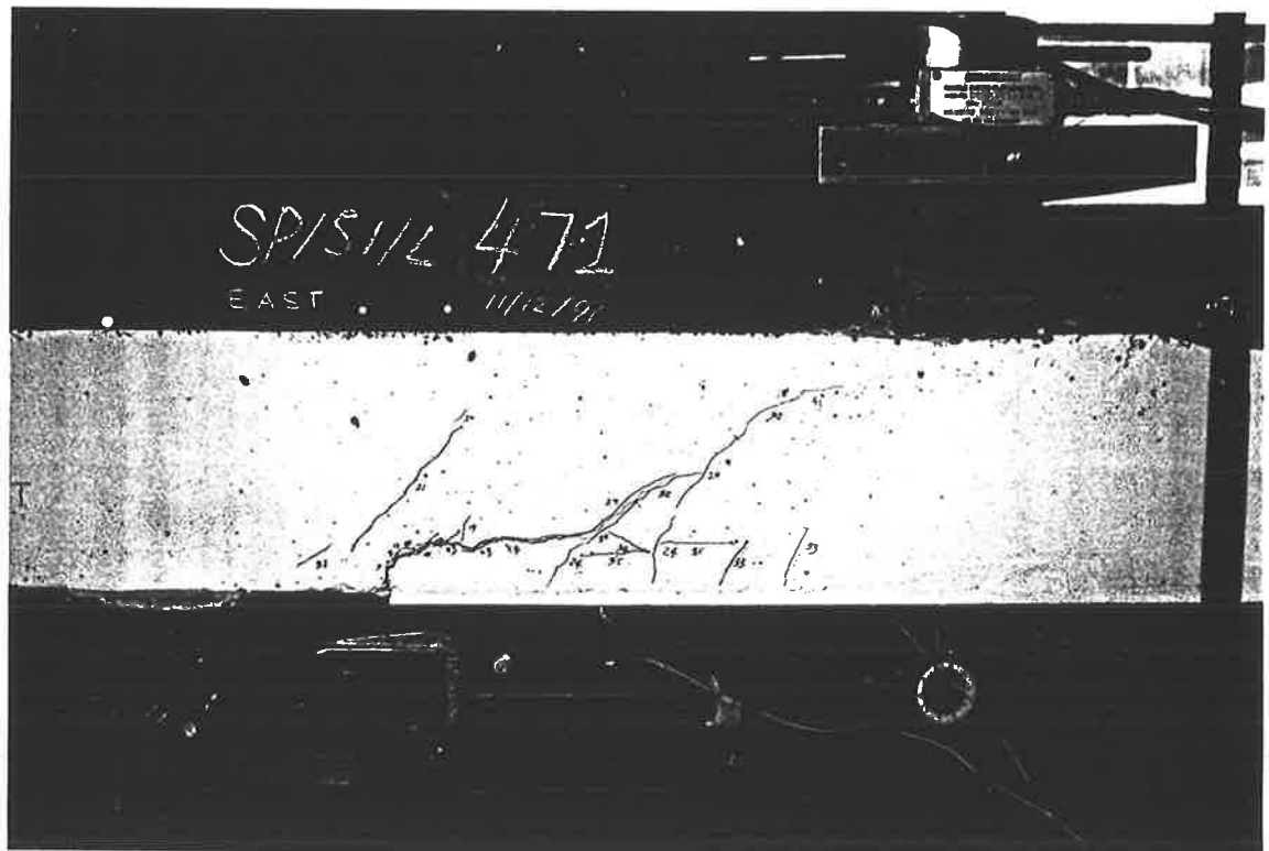
P3-6 Debonding of the soffit plate
