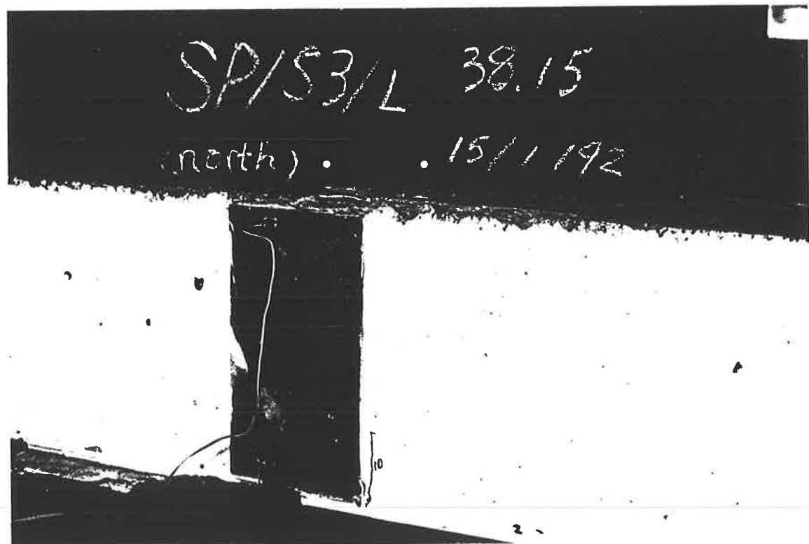
P3-12 Cracks formed along the edge of the side plate in north
