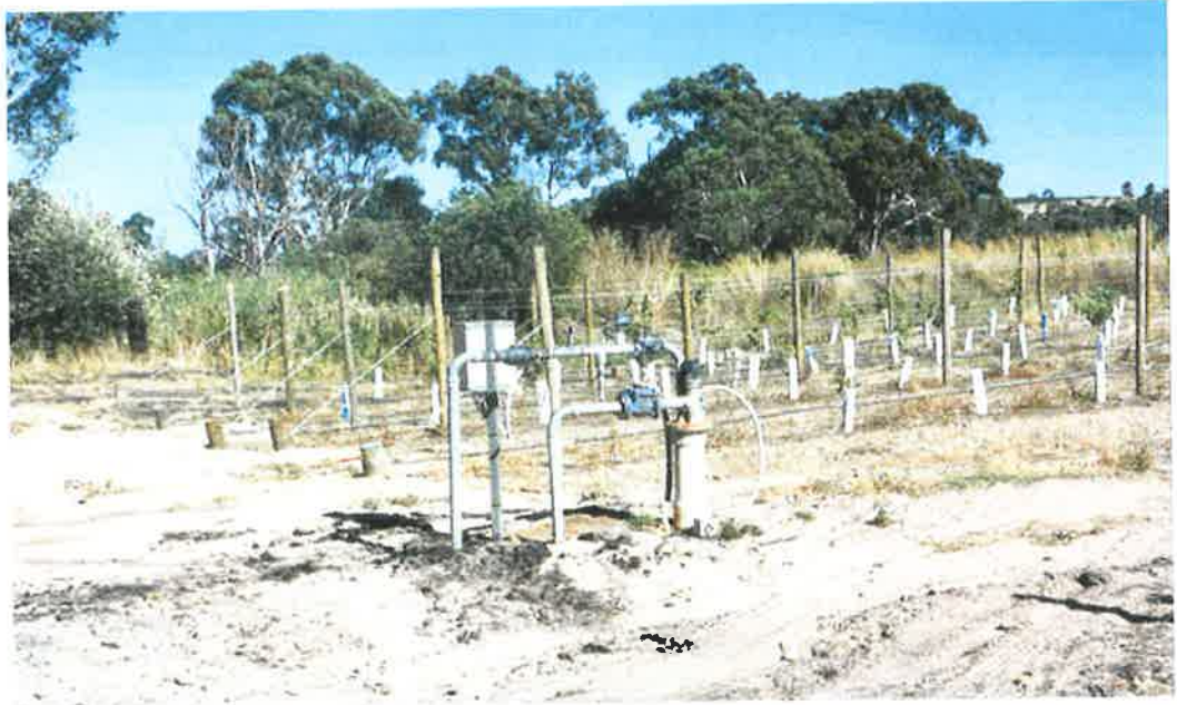
Photo 2.0 Injection and Extraction Well-heads, 'Pedler Divide', McLaren Vale, South Australia
