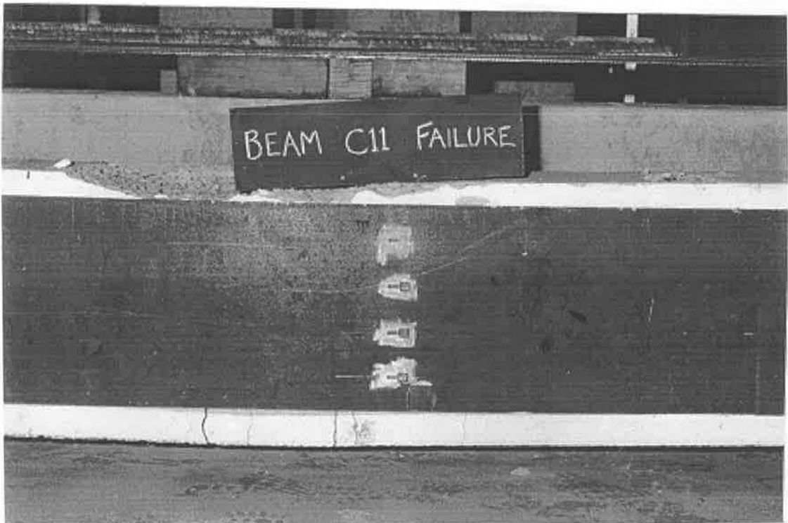
P8.57 Flexural failure of beam C11
