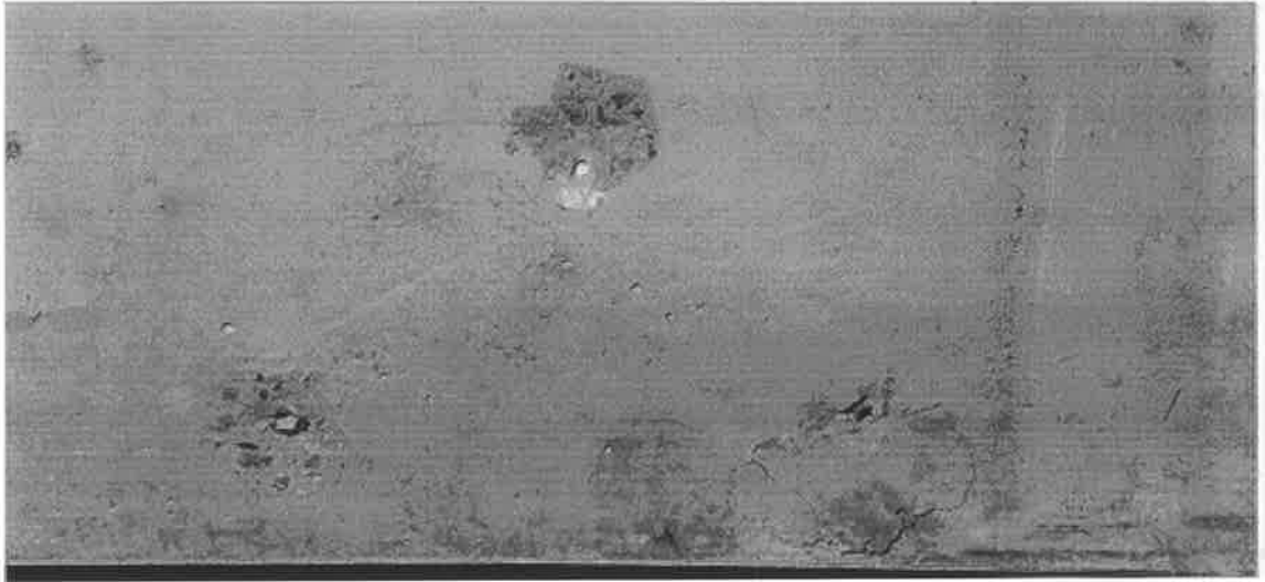
P8.3 Crushing of surrounding concrete of Dynabolt
