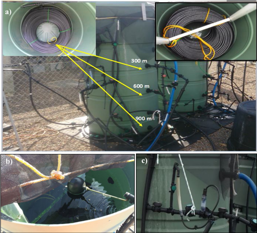
Fig. 2. a) Sampling points on one of the DS's (DS 1 ). Top left photo shows one of the 300 m polyethylene bundles connected to the bottom 'T' section of the tank. Top right photo shows a PVC pipe arrangement to restrain the PE tubing inside the tanks. b) Float ball valve controls the bulk inflow into the DS. c) Pipework configuration to allow measurement of the flow through the DS.
