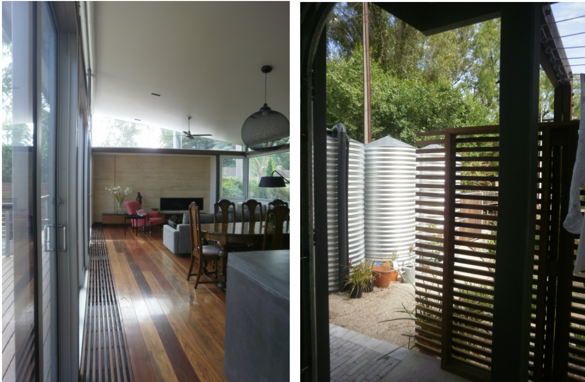
Figure 5.5.1j The hydraulic heating is installed under the floor by heated water pipes coming under the slab (Left) and water tanks (Right) as design features of this contemporary Troppo housing for the moderate climate of Adelaide
