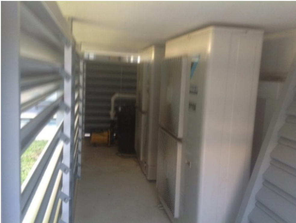
Figure 5.7.1m A fan and a reverse-cycle air-conditioning unit are installed in every room (Top) and the two controlled systems are placed in and covered by a corrugated and shuttered box (Bottom). Photographs were taken by the Howells in 2014.
